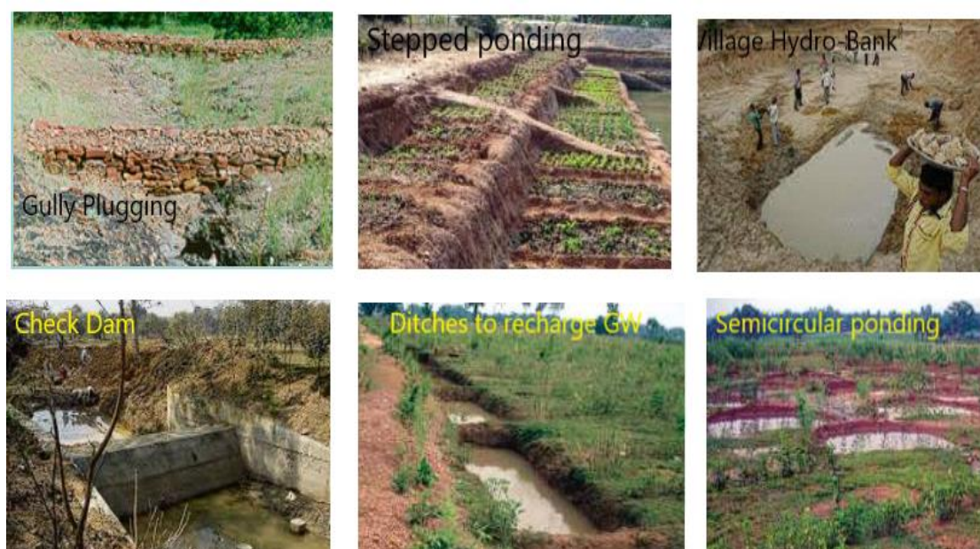
Fig. 10. Some water harvesting structures and groundwater recharging units to combat drought
